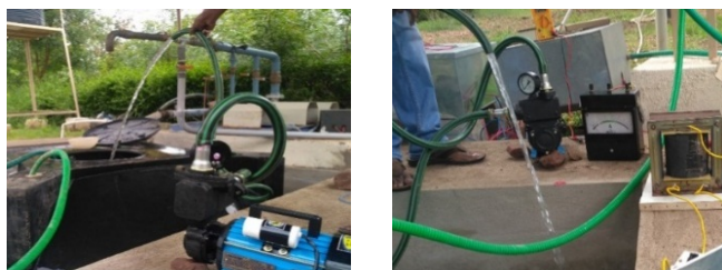
Fig.9: SPV based AC water pumping system-Water Discharge
