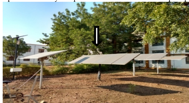
Fig.8: SPV panels installed at Energy Park, BEC, Bagalkot
